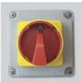
Electrical isolator fitted to fan for security
