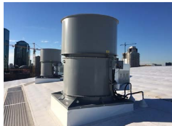
Smoke Emergency Exhaust
