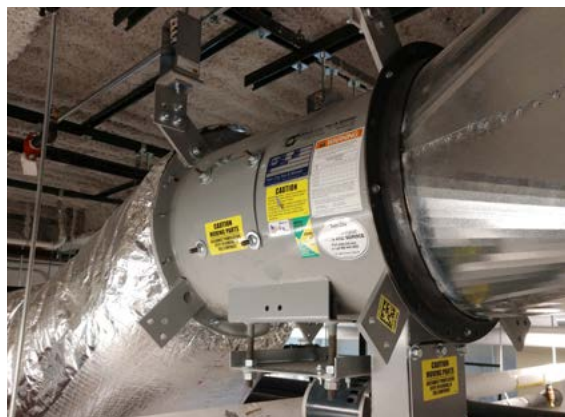
Mechanical Room Exhaust
