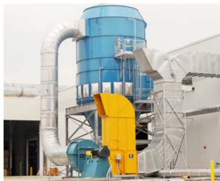
Dust Collection System
