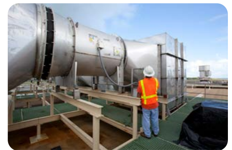
Paint Booth Exhaust
