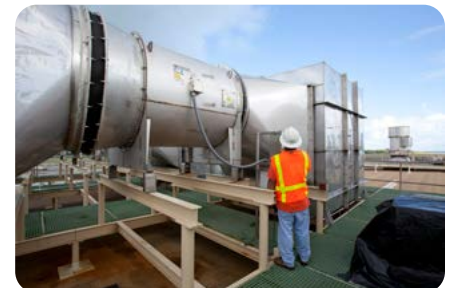
Paint Booth Exhaust
