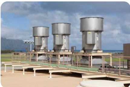
Paint Booth Exhaust
