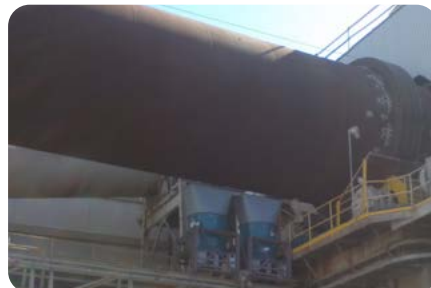
Cement Kiln Cooling
