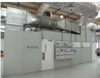
Paint Spray Booth
