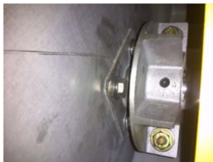
Shaft Cooling Wheel
