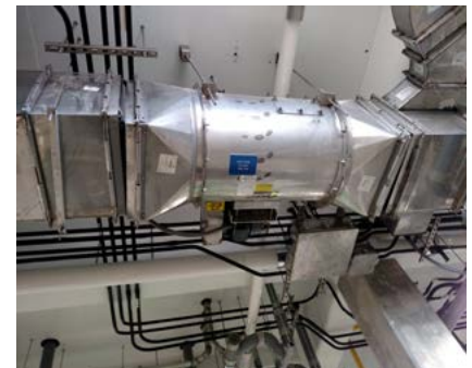
Sewage Treatment Odor Control
